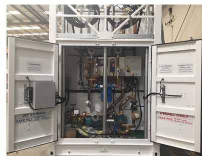
Dual Diesel and insulated DEF chemical resistant tanks
