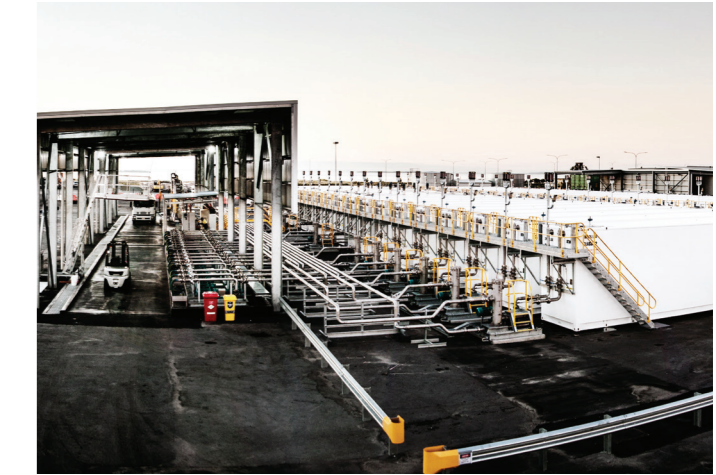
CASTROL BP - 43 x Logitank LSB110 self-bunded tanks, totalling 4.7 million litres of storage for 16 lubricant product
