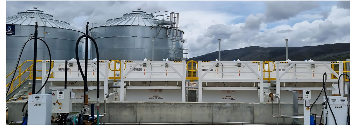
SNOWY HYDRO - Fuelco supplied 4 x LTKO40 (fire-rated) diesel storage tanks
