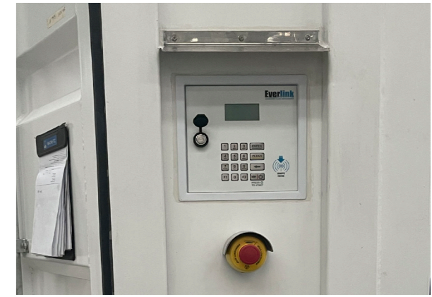
ADDITION OF FUEL MANAGEMENT SYSTEMS
