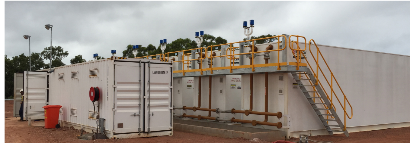
METRO MINING - 600,000L diesel fuel farm. 1x Adblue tank at remote site mine in North Queensland
