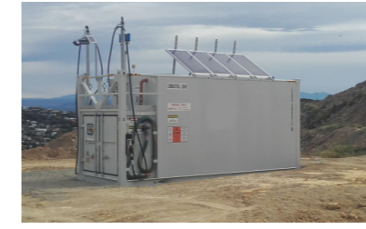
Solar Tank for Farming Client New Zealand
