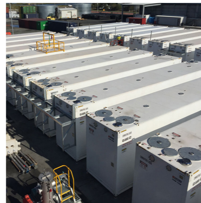
WESTERN TURNER PROJECT - 11 x Classic Tanks Diesel
