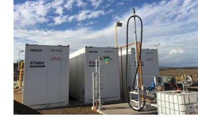
Mine Site Refuelling Facility Australia
