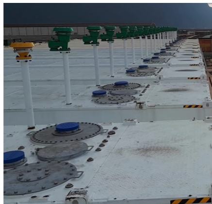
SOCOTTRA 5,000,000L fuel storage
