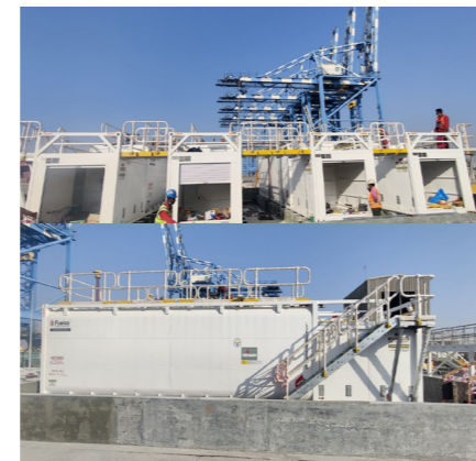
Fuel Depot for a Port in UAE 4xLTKB 47 – 2 hours Fire rated tank. Capacity – 47,000L GFL per tank
