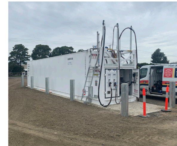
COMBO (DIESEL & ADBLUE) TANKS UNMANNED FUEL STATION, AUSTRALIA
