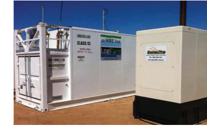
Back-up for Power Generation Australia
