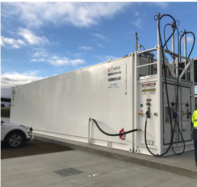
Dual Diesel and insulated DEF chemical resistant tanks
