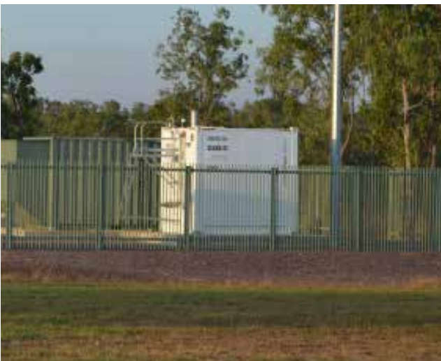
Pictured refuelling a pumping station
